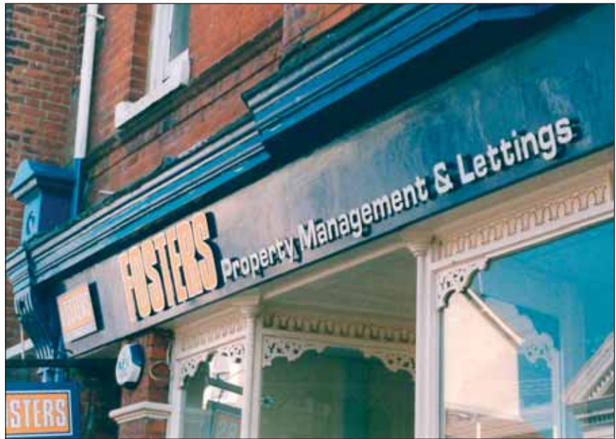
Shop signboard on the High Street to show Victorian deepening of fascia to allow more room for advertising, with a more elaborate cornice above.
