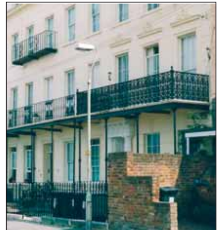
Close up view of further section of Terrace to west showing continuous iron balcony.
