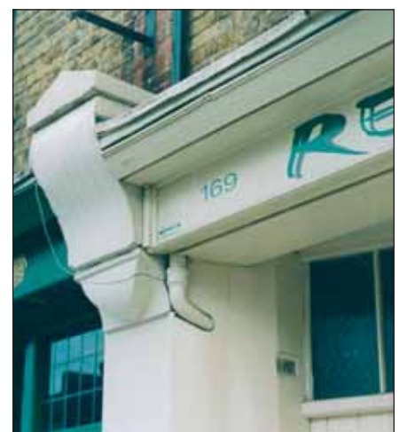
Very simplified later console bracket, signboard and cornice. The sloping part of the cornice is the front of the blind box for a canvas roller blind.
